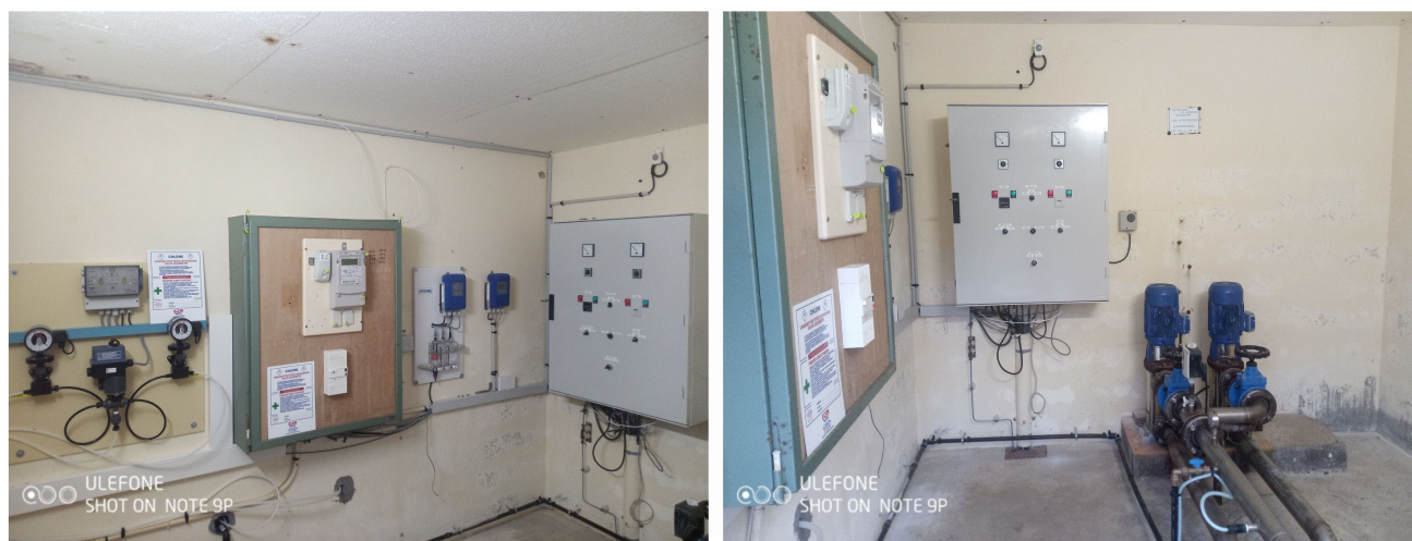
Figure 6 : station de pompage Rousson.
